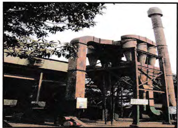
Photograph 6: Dust Extraction System at Crushing Plant
