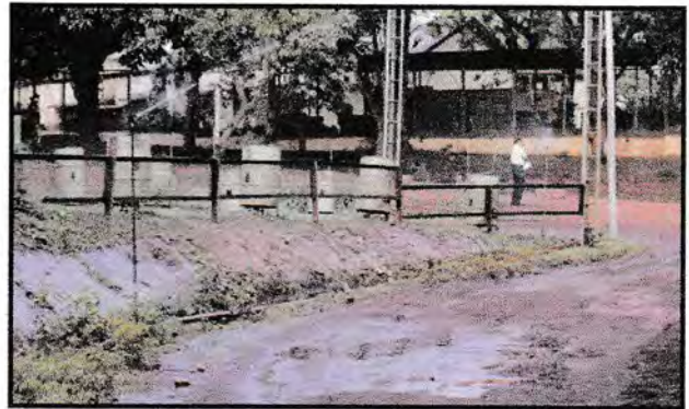
Photograph 4: Permanent Sprinklers at OHP
