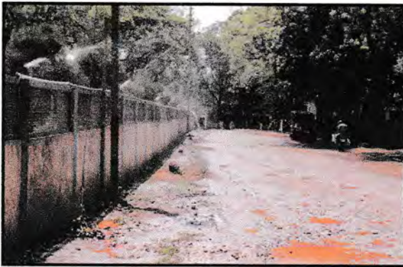
Photograph 3: Permanent Road Sprinklers in Township
