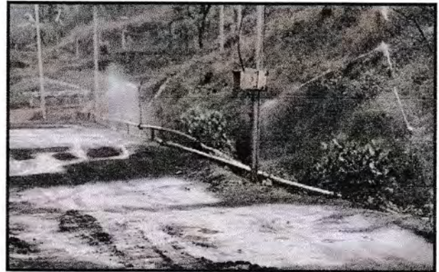
Photograph 2: Permanent Road Sprinklers in Mines
