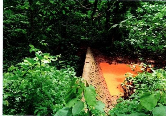
CHECK DAM SHOWING SILT CONTROL IN MONSOON
