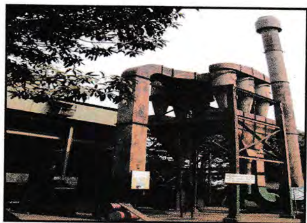
Photograph 6: Dust Extraction System at Crushing Plant
