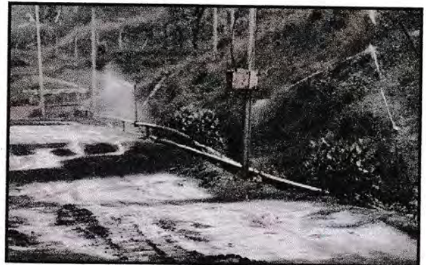
Photograph 2: Permanent Road Sprinklers in Mines
