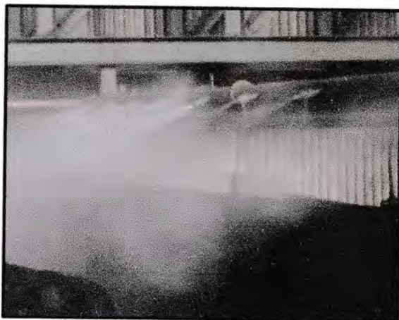
Photograph 5: Dry Fog Dust Suppression System at Hopper
