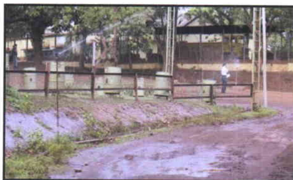
Photograph 4: Permanent Sprinklers at OHP
