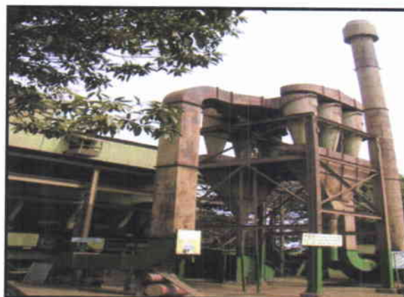
Photograph 6: Dust Extraction System at Crushing Plant
