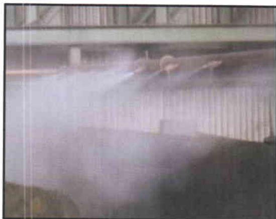
Photograph 5: Dry Fog Dust Suppression System at Hopper
