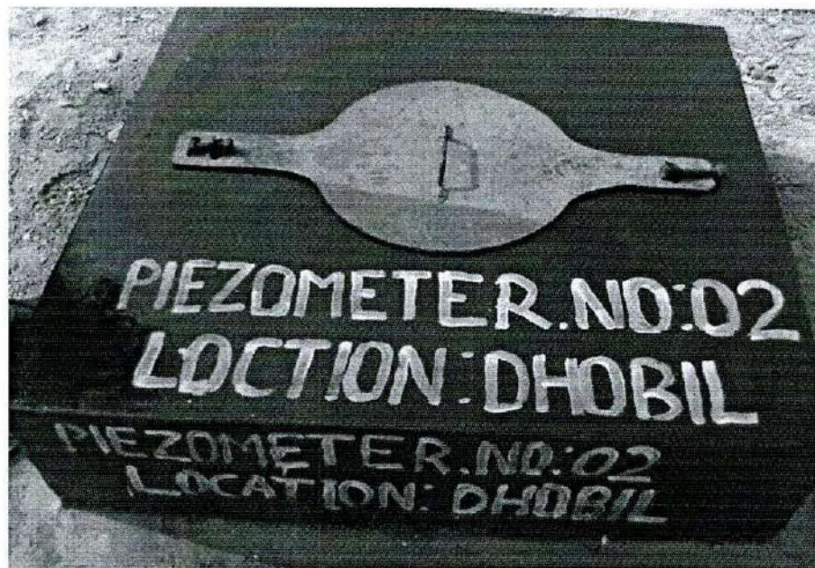
2. Piezometer at Dhobil Village
