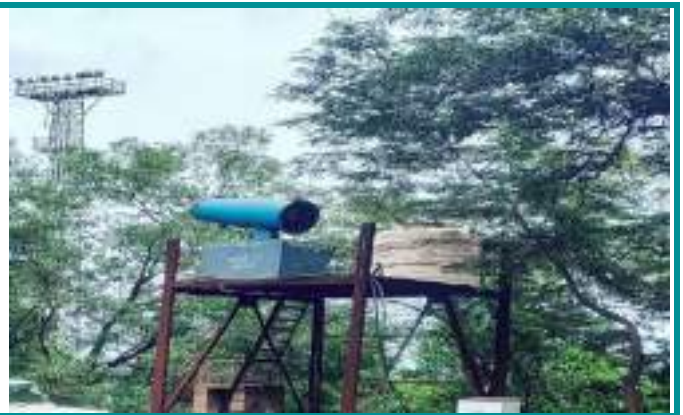
Rotating Fog Canon Installed at SSP
