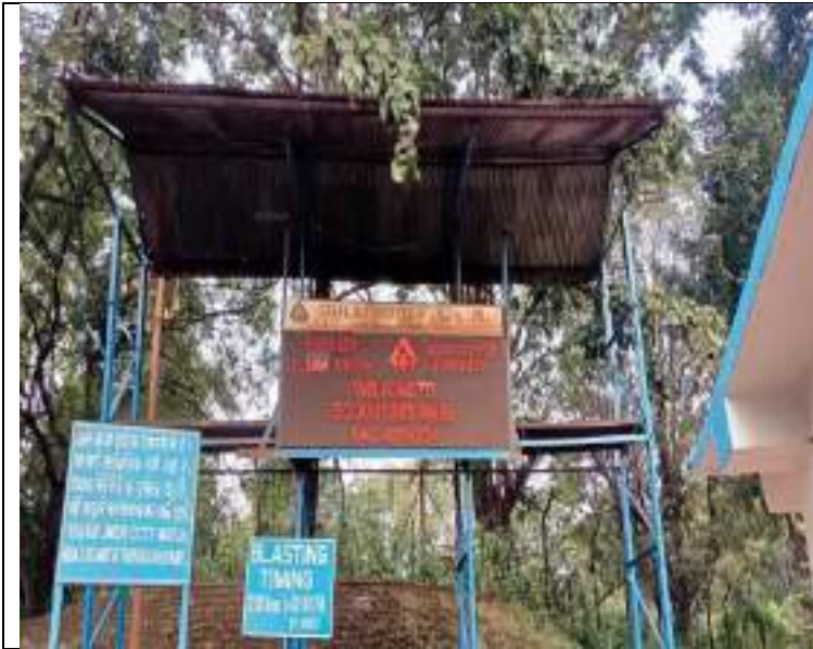
Electronic Display Board Installed at Mines Entry Gate
